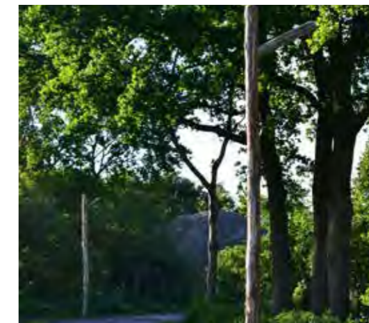
Natural looking street lamps to maintain the landscape aesthetic, directional as to not disturb bats.
